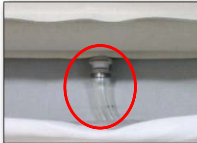
Locate Hose Connection(s) at Head of Bed
